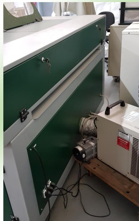
Vista Traseira (Chiller, compressor)
